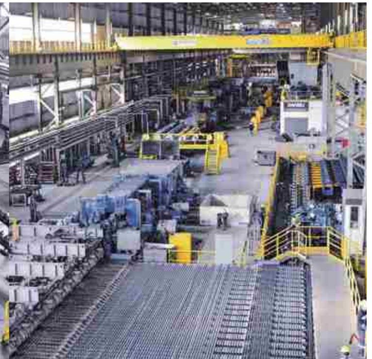
Finishing services and rolling mill overview
