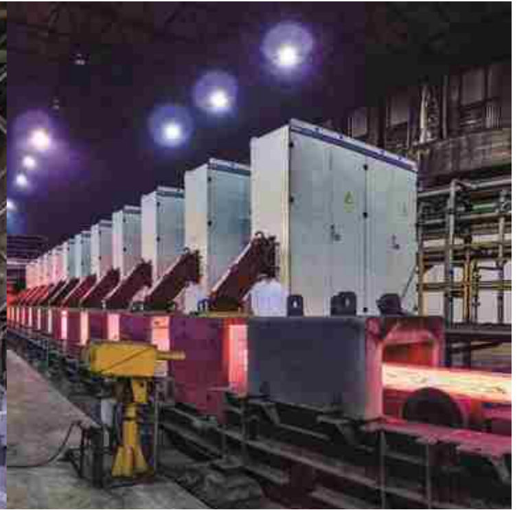
Induction line made of 20 Q-Heat units
