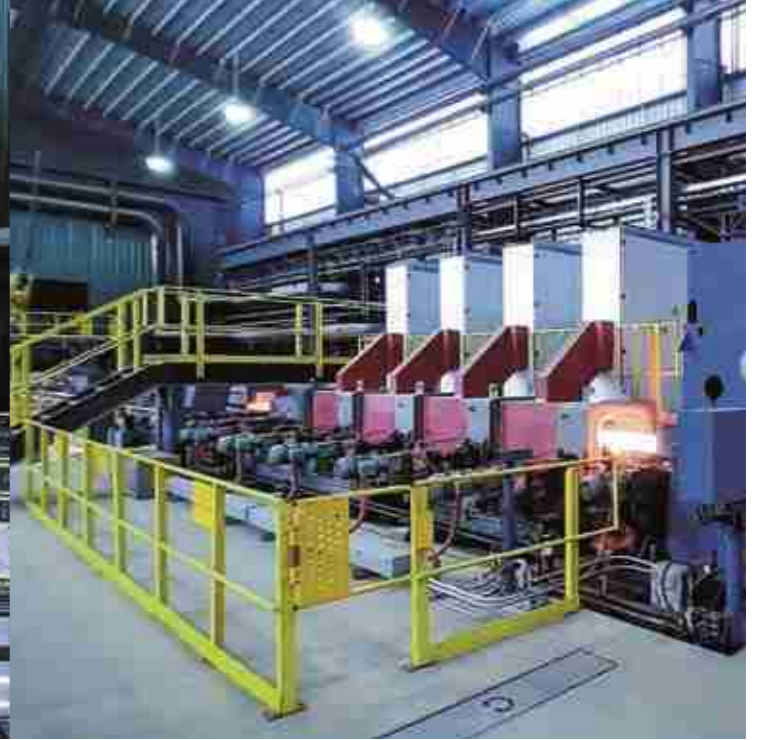
Q-Heat induction heating system (4x1 MW)
