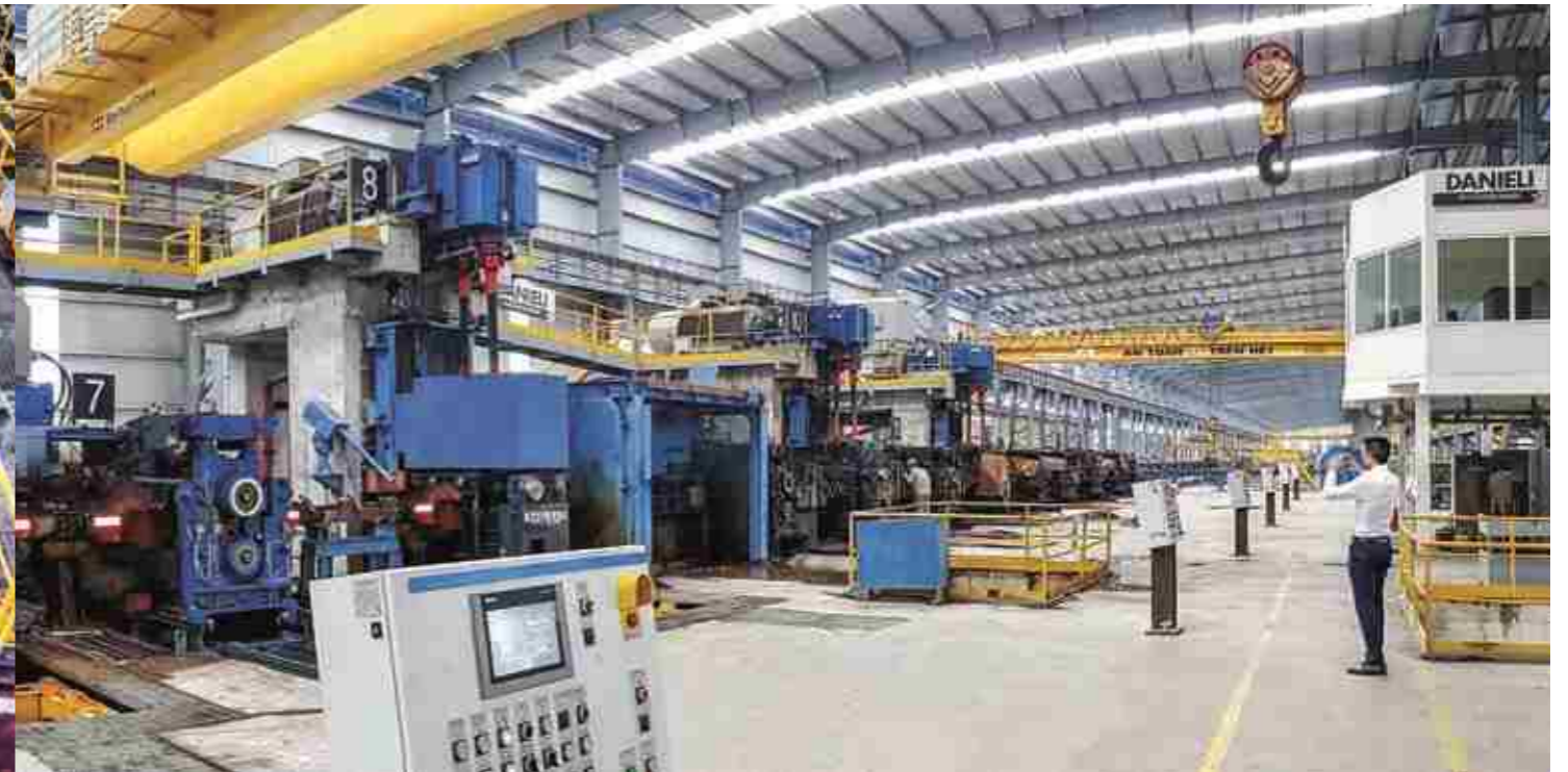
4+4+4 housingless stand mill followed by 2x 4 ESS cantilever stands and a 10-pass finishing block
