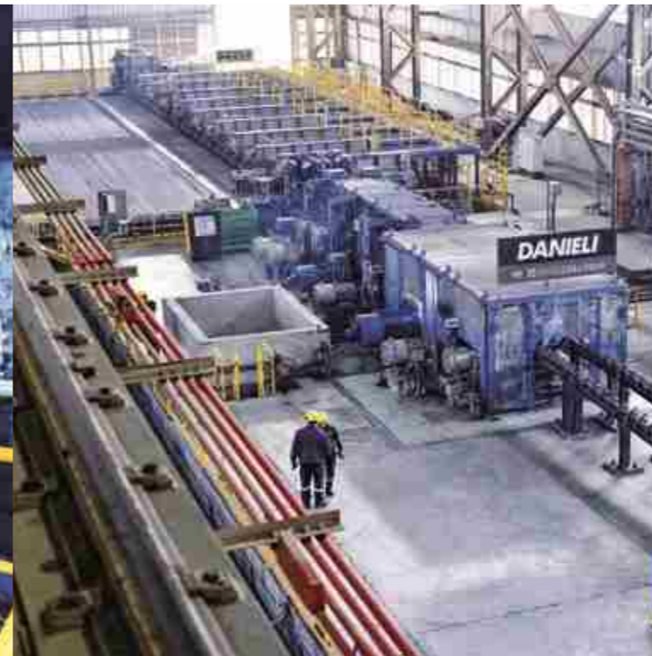
Cut-to-length area preceding DRB building unit
